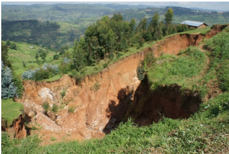
Fig. 5.8: Large gully at the edge of the Gihembe Refugee Camp caused by soil erosion
