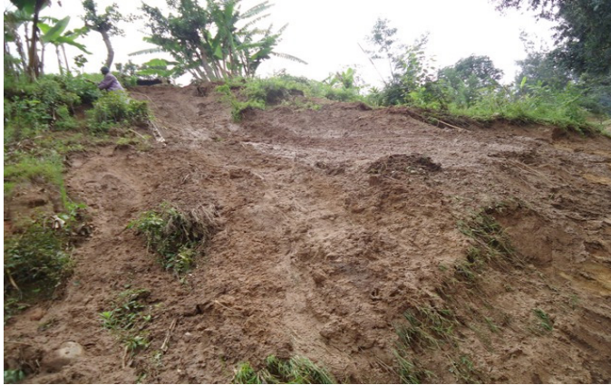
Fig 5.5: Soil erosion on a slope
