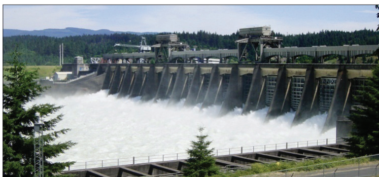
Figure 6.14: Hydroelectric power station
