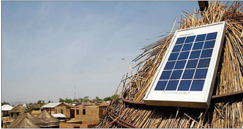
Figure 6.12: Israel's Energiya Global is behind a new solar project in Rwanda
