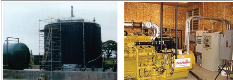
Figure 6.7: Burning landfill and digester gas to make power
