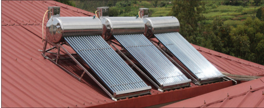
Figure 6.13: In Rusizi, solar heating panels on a roof of a house
