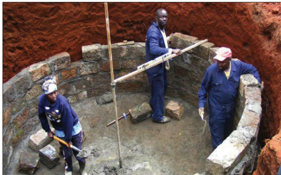
Figure 6.8: Construction works of the digester chamber for a fixed dome bio-gas plant. Biogas will play a key role in reducing pressure on the country's forests
