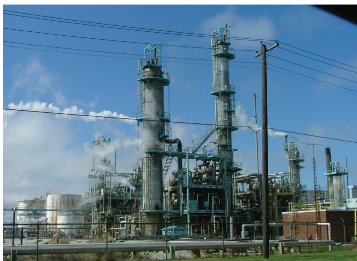
Fig 1.6. An Oil Refinery
