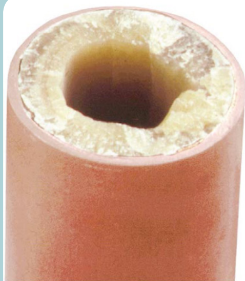
Pipe with limescale
