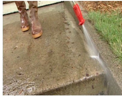
Cemented floor (floor covered by the carpet)
