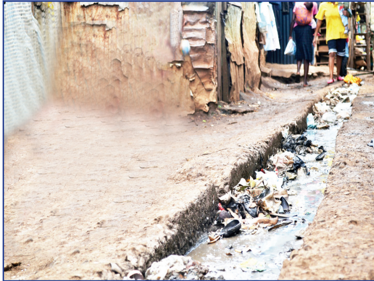
Figure 4.12: Open sewage and sanitation conditions.
