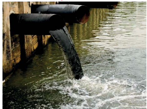
Fig 10.6 Industrial waste being dumped in a water source (This should be discouraged)
